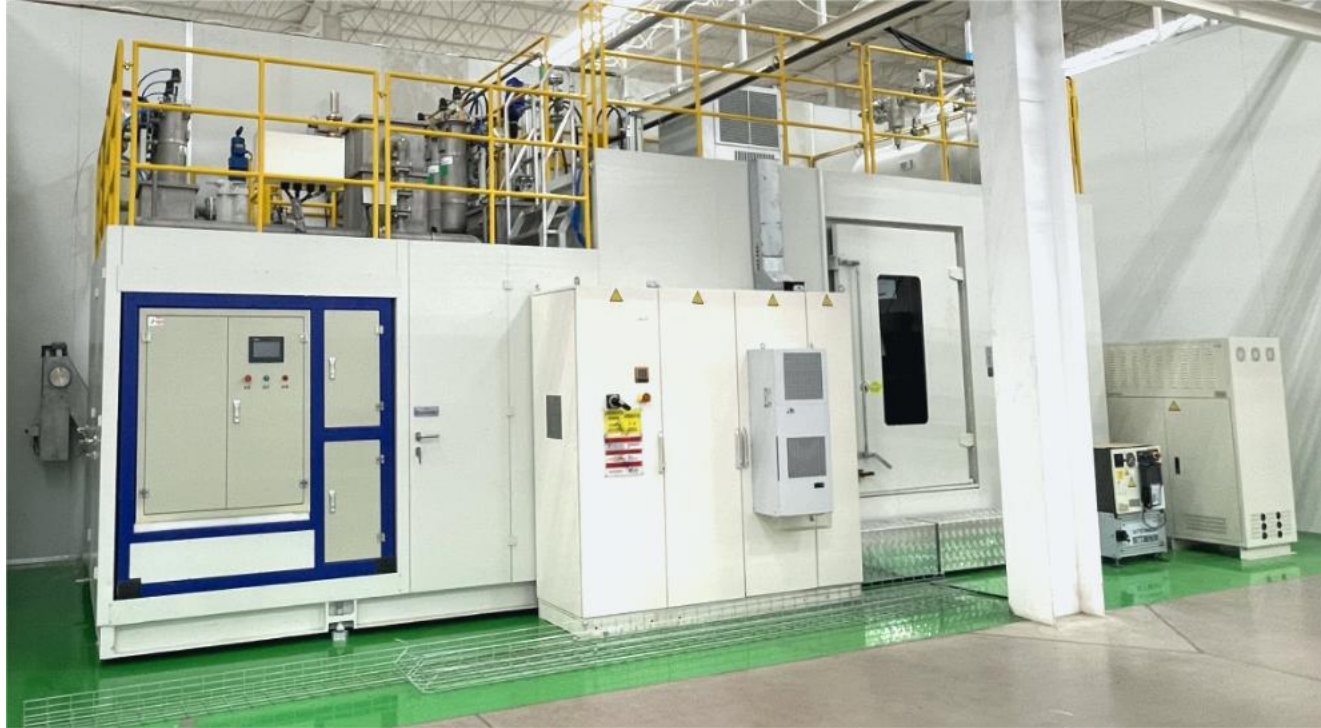
Dedicated High Pressure Cleaning Line for Transmission Case
